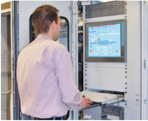
RST software engineer performing final acceptance of the visualisation software for a gas turbine
