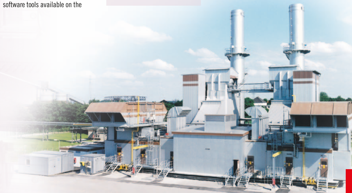
Control and visualisation system for two gas turbines running a generator with one downstream waste-heat boiler for each gas turbine
